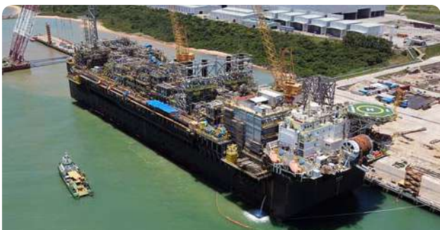
P-71 FPSO undergoing modification, integration and topside works in our Brazil yard for deployment to the Itapu Field
